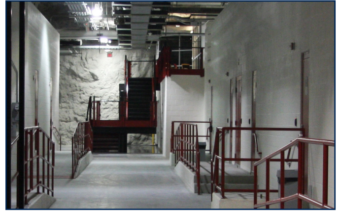
SpringNet Underground has 60,000 sqft of co-location space in Springfield. The “building in a building” concept currently houses several companies with plans to expand.
