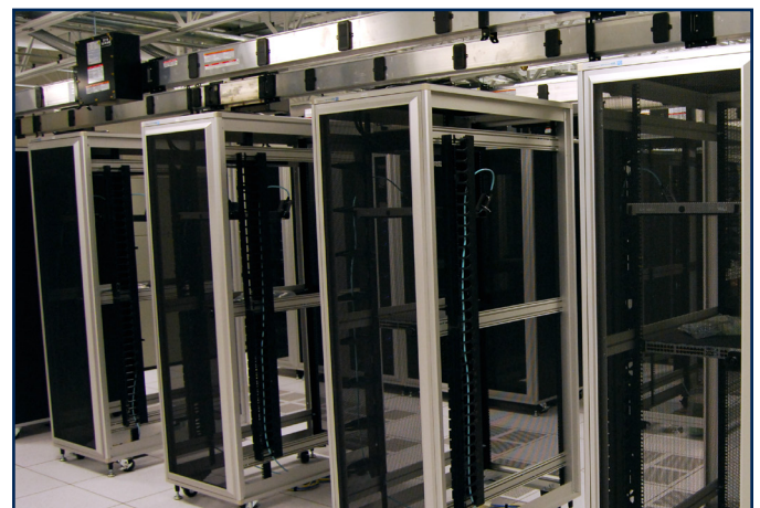
A green benefit of being underground is the natural year round air temperature of 60 - 64 degrees Fahrenheit which serves to “naturally” harden the facility and helps provide the ideal computing environment.
